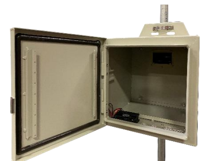
Enclosure interior without batteries or controller
