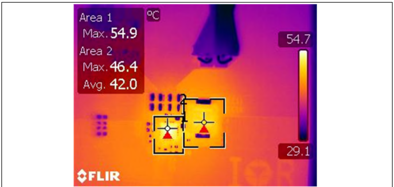
Figure 24 Thermal Image of the board at 3 A load IR3883 = 55 °C, L= 46 °C, Amb = 25 °C
